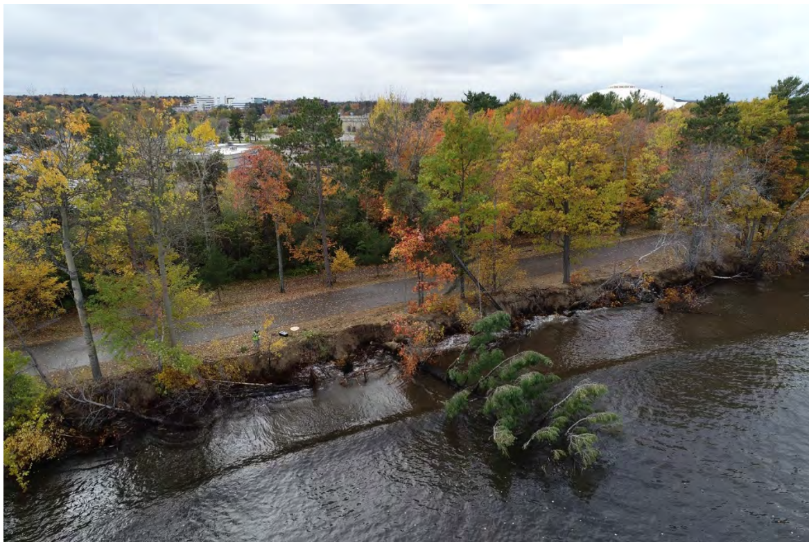
Photo 3. Addition shoreline damage that occurred during the fall of 2019 south of the project area.
