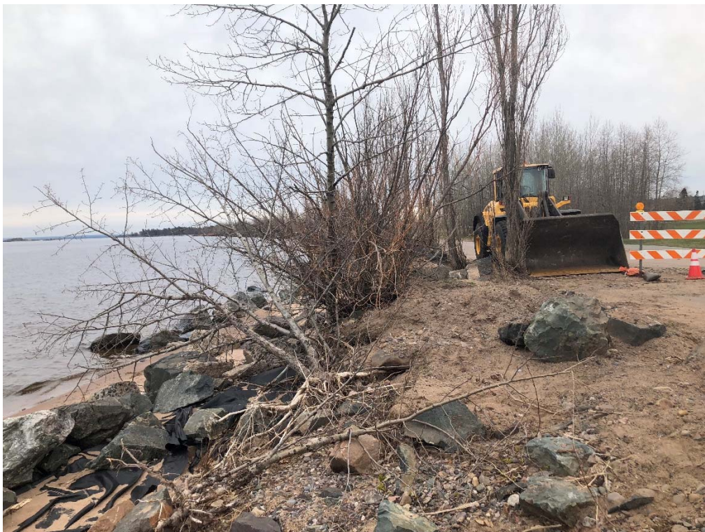
Photo 11. Looking south at shoreline damage adjacent to Lakeshore Boulevard. Note the road is very close to the lake in this area and is frequently overtopped by waves.
